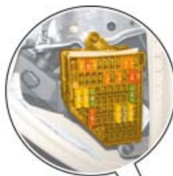
Fuse box, right of dash panel
